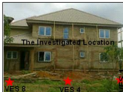
Figure 2b: Location of the VES stations and the patched cracks in the building.
