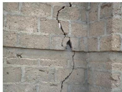
Figure 2c: The cracks notice at the Eastern fence that separates the building from another house.
