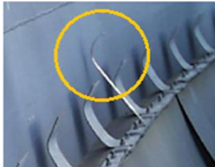
Figure 3: Shunt Not Making Contact with the Tank Copyright: Lightning Eliminators and Consultants, Inc. 2012
