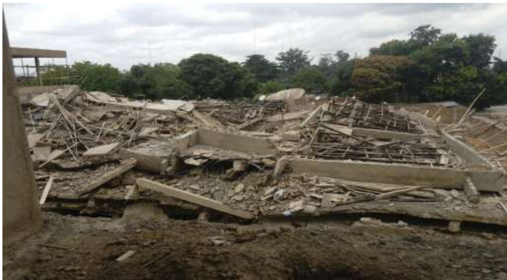
Figure 1 The building unit that collapsed (Aremu, 2018).
