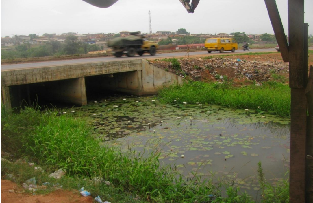
PLATE V River Atuwara upper boundary at Owode – Ijako along Lagos Abeokuta Expressway
