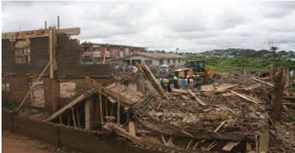
Figure 1 Rubble of a church building that collapsed in Ibadan, Nigeria [24].
