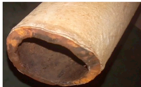
Fig. 4. Section of the Flow Line with Large Internal Corrosion.
