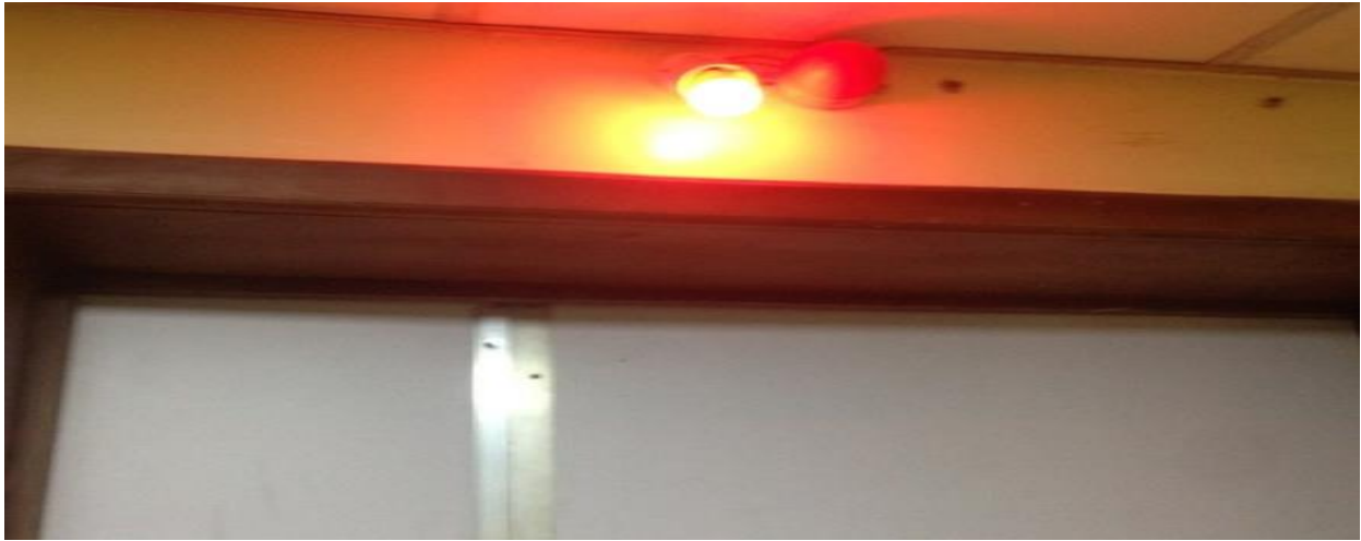
Plate 12: View showing danger signs on the entrance door leading into the radiology room.
