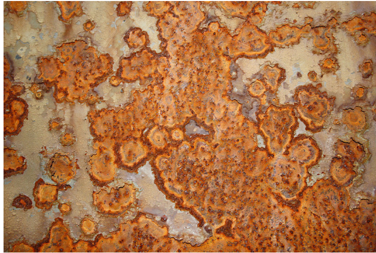
Figure 1: metallic corrosion caused by atmospheric aerosols
