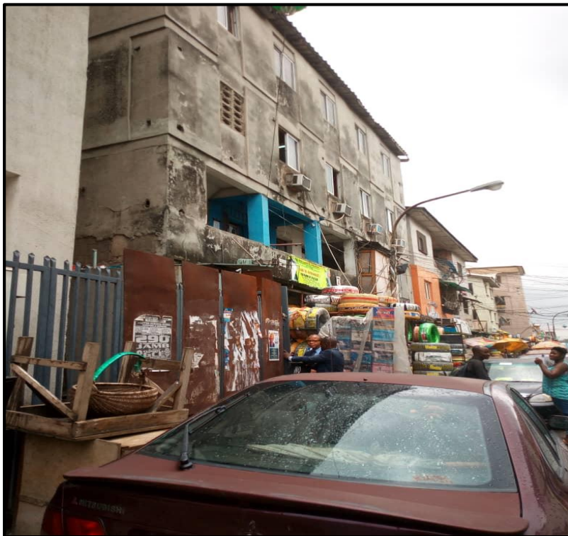
Figure 3: The effect of the climate on the plastering material on the wall of the building Source: Authors research.
