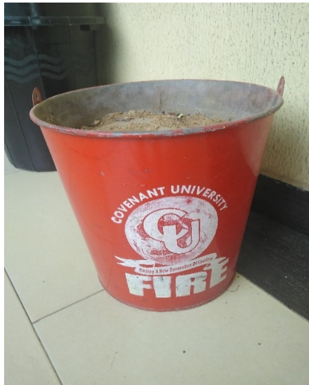
Figure 6. Fire bucket positioned along a corridor
