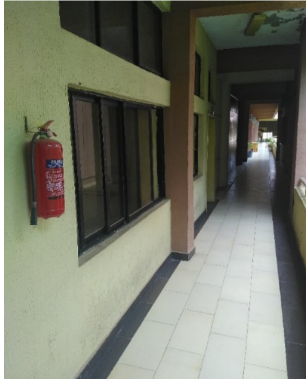
Figure 5. Fire Extinguisher hung along a corridor
