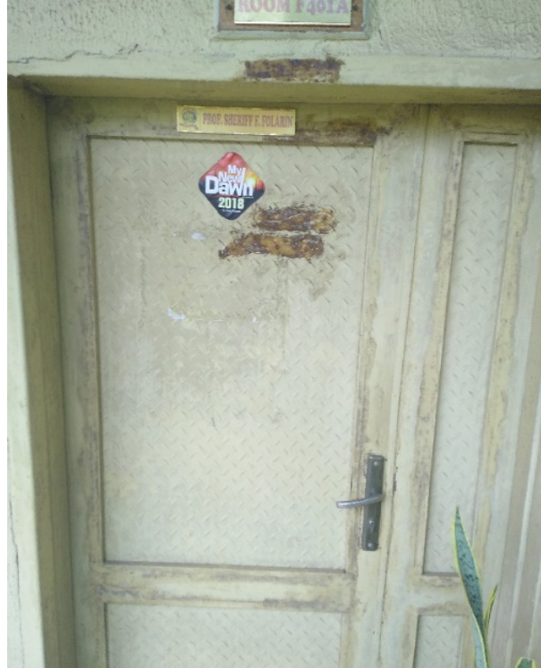
Figure 7. Non-Fire Resistant Door
