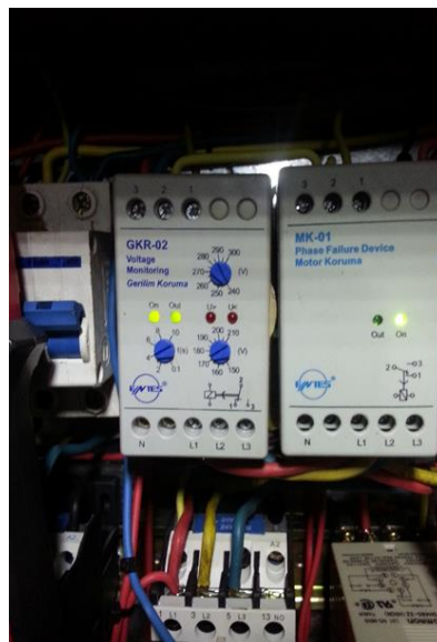
Figure 7. Voltage monitor indicating normal voltage input after adjustment of the lower limit.
