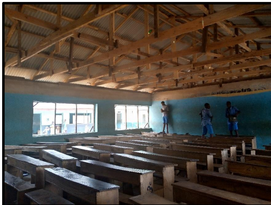
Plate 4.45 View of non-existent ceiling
