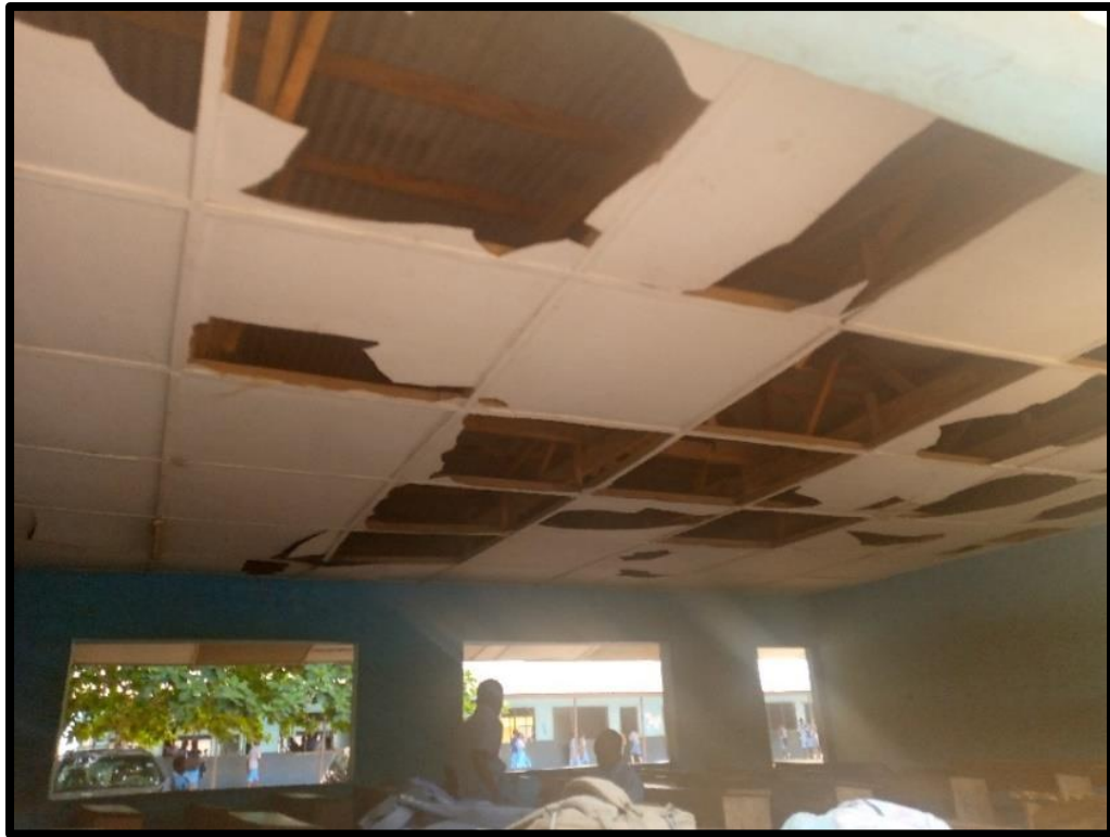
Plate 4.44 View of dilapidated ceiling
