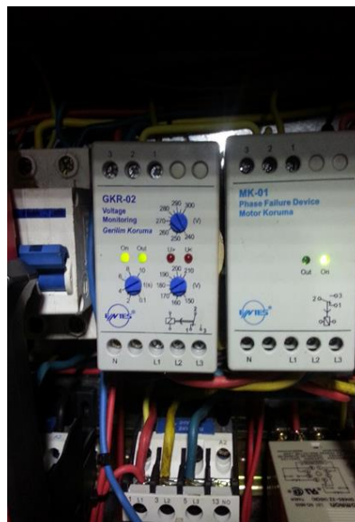
Figure 7. Voltage monitor indicating normal voltage input after adjustment of the lower limit.
