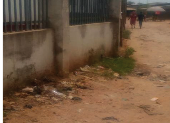
Figure 2. A greywater outlet pipe from Grocery Bazeer mall opening into the adjacent road
