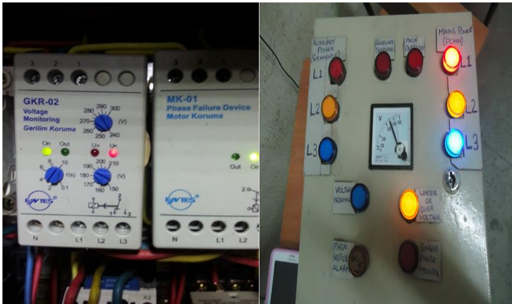
Figure 6. Voltage monitor showing an under-voltage input and indicator panel
