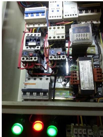
Figure 4. All bulbs on, indicating complete Three-phase supply
