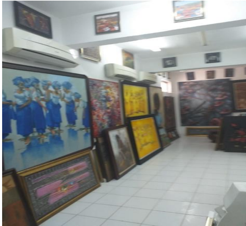
Plate 4.9 Air conditioning units used in Nike art gallery, Lekki, Lagos Source: Author's fieldwork (2021)
