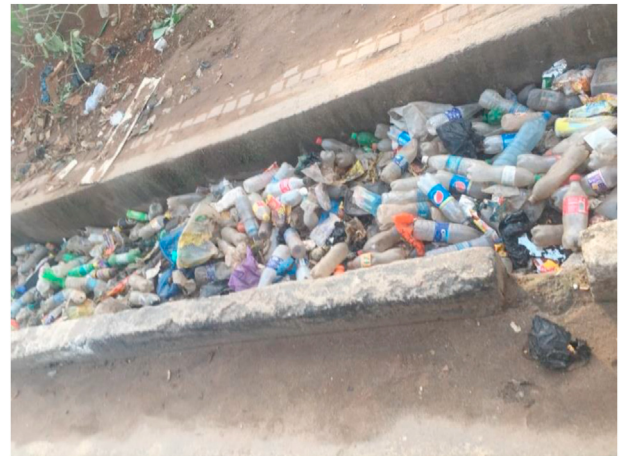
Figure 1. Plastic waste blocking drains.
