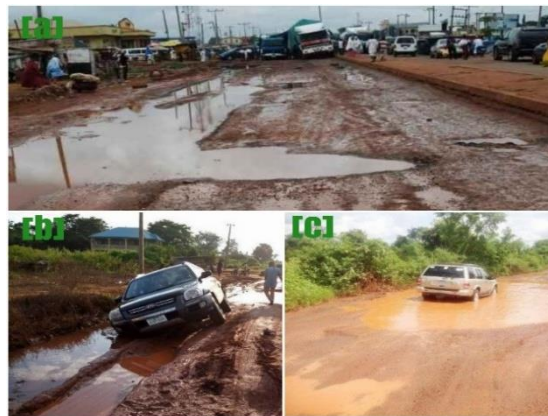
Figure 1. (a) Kaduna – Abuja road (North Central Nigeria), (b) Otukpa-Otukpo Markurdi, (North Central Nigeria), (c) Enugu – Awka - Onitsha road (Eastern Nigeria)
