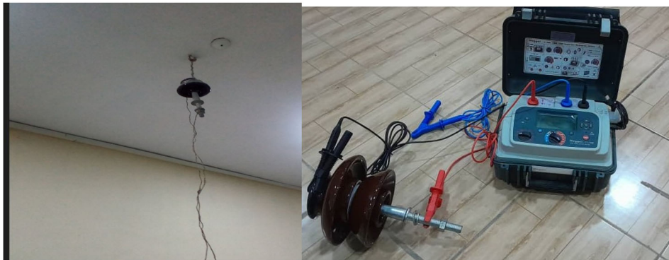
Figure 5. The test bed used for the insulation testing using Megger S1-1568 15 kV insulation tester.
