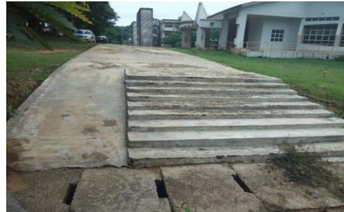
Plate 9. Main Access point to Main walkway servicing all the building blocks that makes up the Faculty of Environmental Science Building
