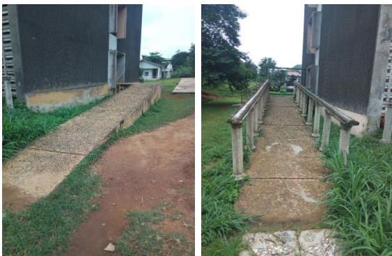
Plate 8. Ramps provided for the Right and Left Wing of the Building Blocks Respectively
