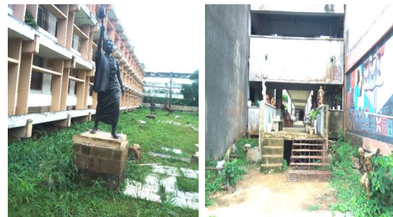
Plate 12. External Areas showing absence of walkway and ramps
