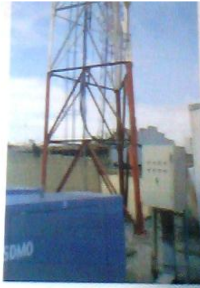
Plate 1: Picture of typical base transceiver station.
