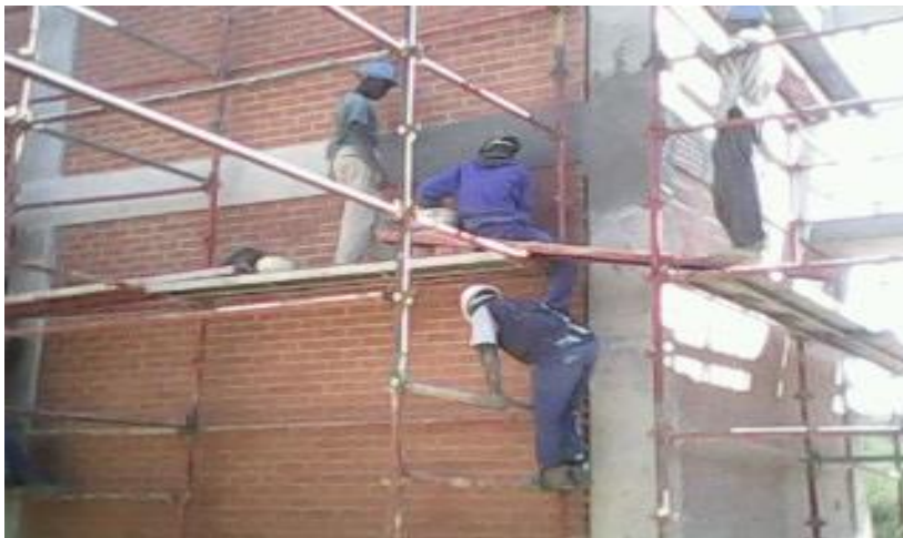
Figure 1 Subcontractor`s workers without safety belt while carrying out their task Note: Photo taking by researcher – 3rd April 2012 in Pretoria site.
