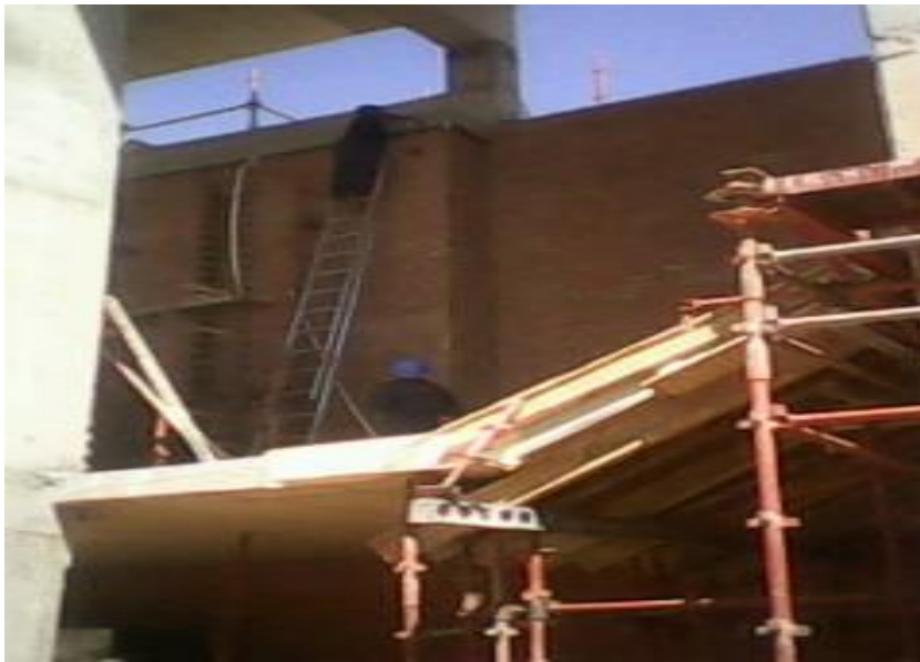
Figure 2 Worker Attitude to safety harness (non-use of safety belt on the ladder) (Photo taking by researcher– 5th July 2012 in centurion site).
