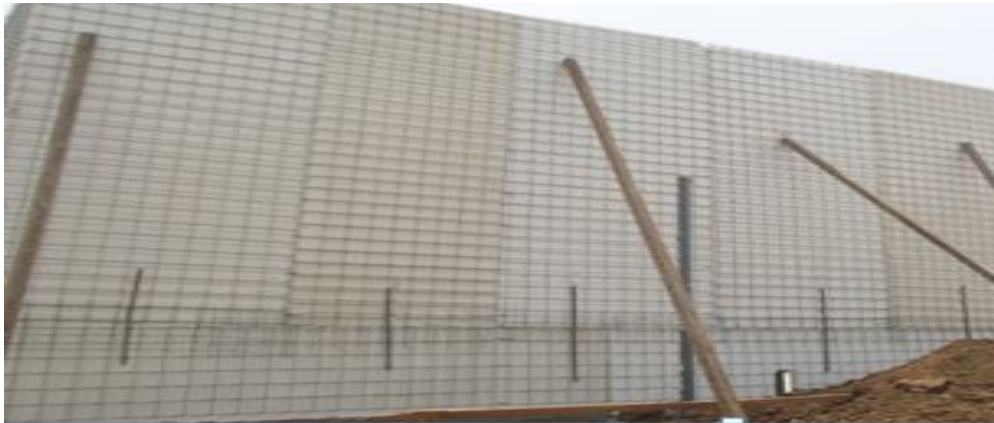
Figure 6: Polystyrene meshed panels used as wall panels on a building site in Maitama, Abuja
