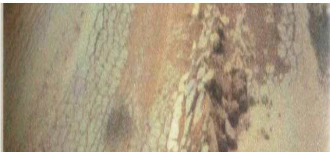
Figure 1 Longitudinal cracks on a highway pavement at oniyale,ifo locality
