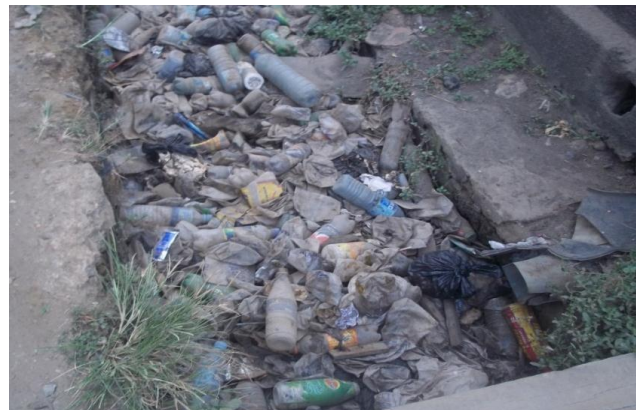
Fig. 8 Indiscriminate dumping of waste in drainage
