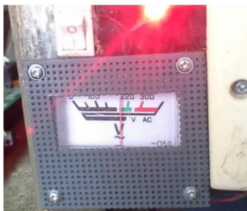
Figure 13: Output Voltage Reading of the No-Load Test
